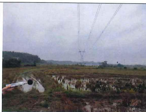
220kV 漳唐线#28~#29 杆塔间声环境衰减断面
